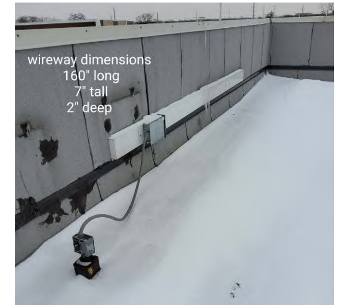
Reuse the raceway behind the wall
