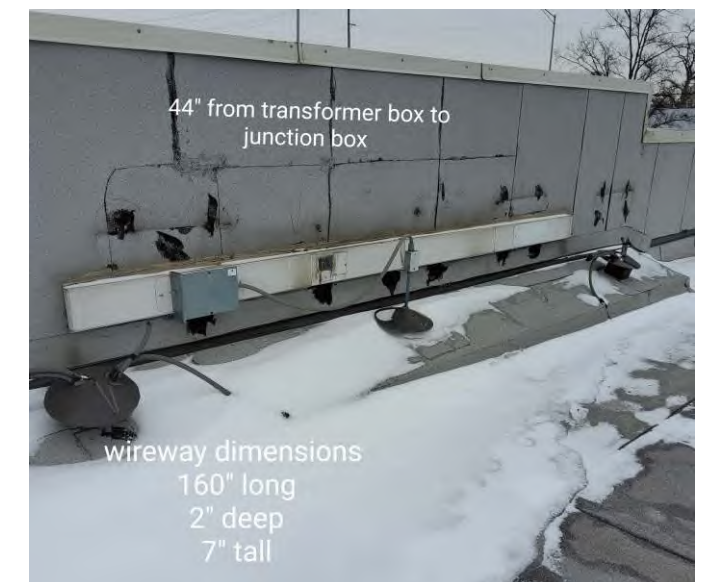
Reuse the raceway behind the wall
