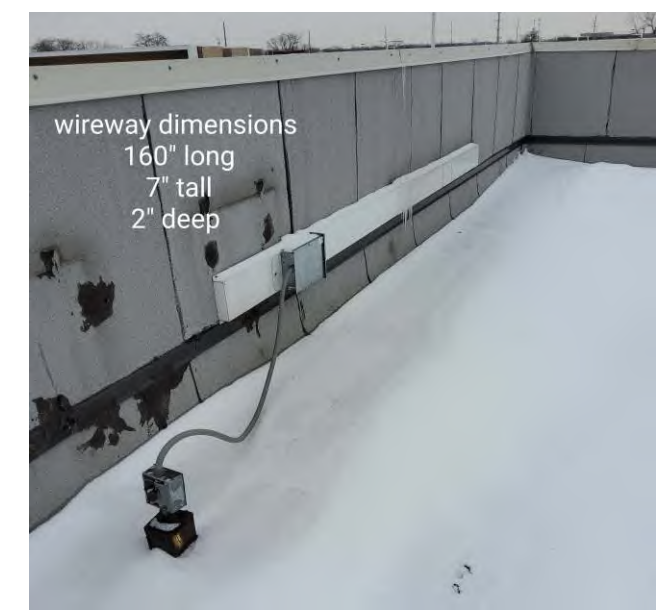
Reuse the raceway behind the wall
