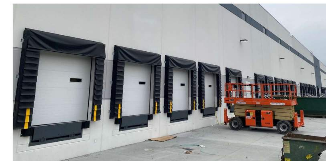
17 OVERHEAD DOCK DOORS
