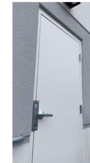
9 INSULATED MAN DOOR
