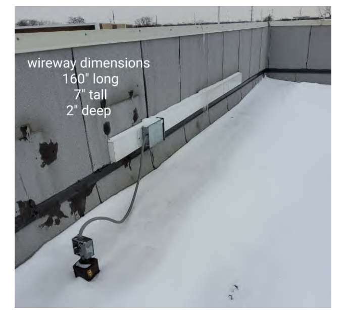
Reuse the raceway behind the wall
