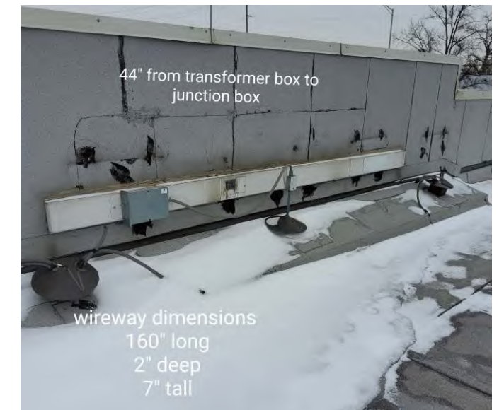
Reuse the raceway behind the wall
