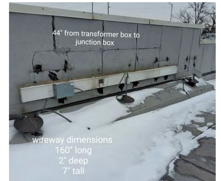
Reuse the raceway behind the wall
