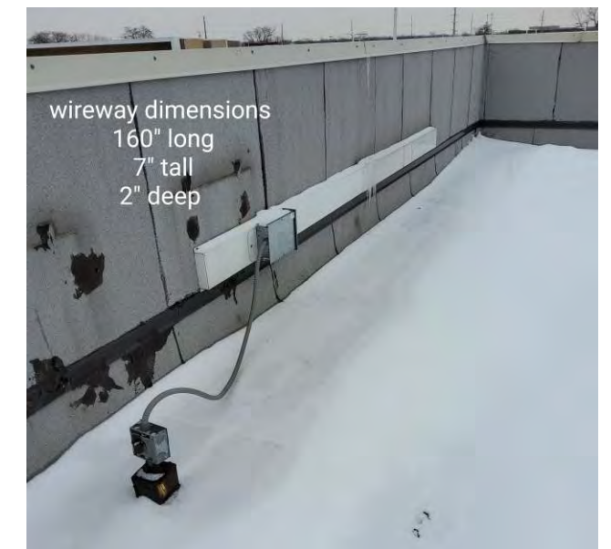
Reuse the raceway behind the wall
