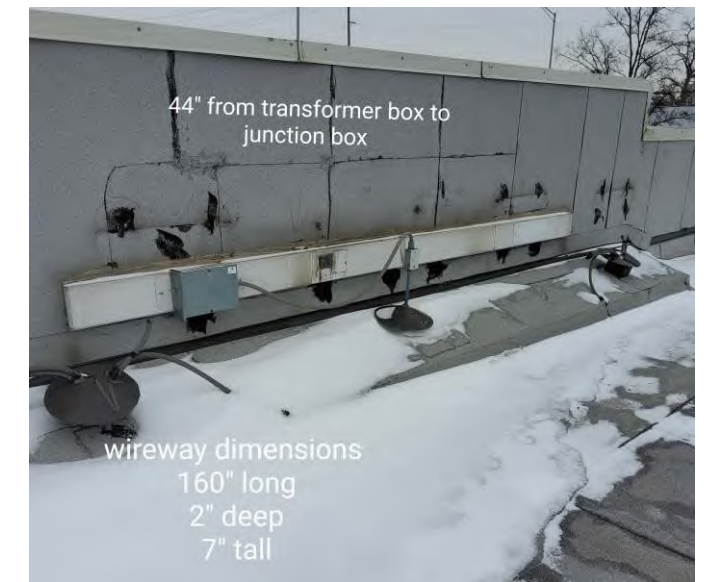
Reuse the raceway behind the wall
